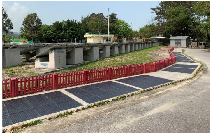
Steppable PV Panels at SHWSTW (Trial)
