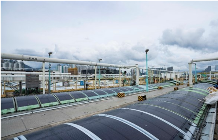
Thin Film PV Panels on curved sedimentation tank covers at SCISTW
